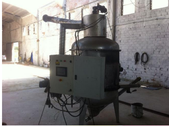
Figure 3. Turbulent combustion incinerator at working place.
